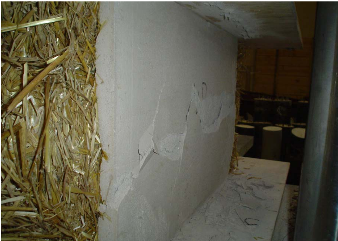
Figure 12: Typical failure of on-edge, plastered straw bale.
